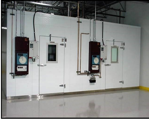
Temperature-Humidity Stability Rooms
